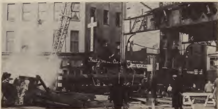
The light comes through as the Third Avenue Elevated is demolished from Brooklyn Bridge to Chatham Square.
